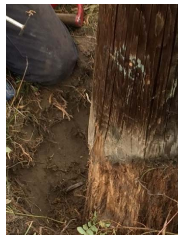
Figure 6-3: Close-up of external decay to be removed in preparation for external treatment
